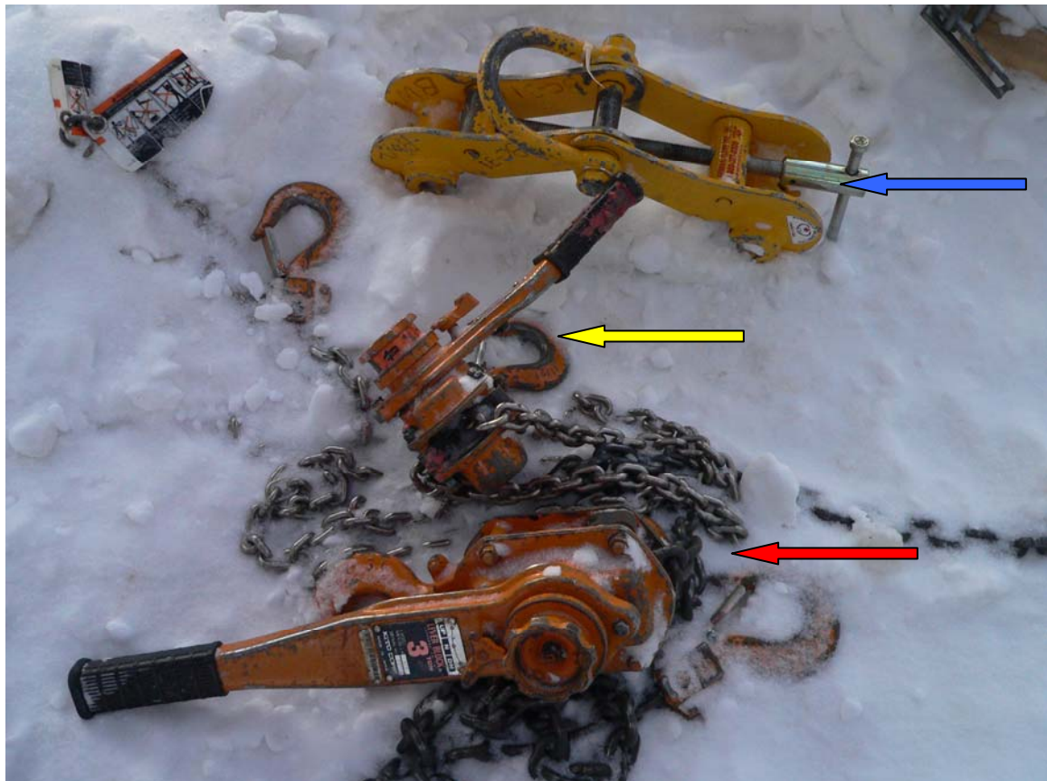
Photograph #2 Shows the beam clamp (Blue arrow), 1 1/2 Ton (yellow arrow) and 3 Ton come-a-long (red arrow) used to tug the pipe spool. The last position of the come-a-longs was disturbed to provide emergency assistance to the worker.
