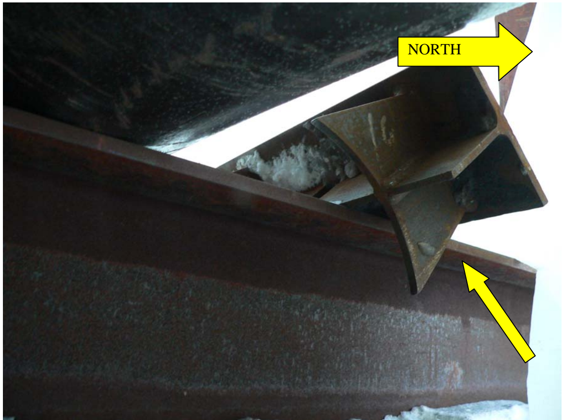
Photograph # 7 Shows the pipe spool dislodged from the cradle of the pipe shoe (yellow arrow). The pipe spool had tipped to the South.
