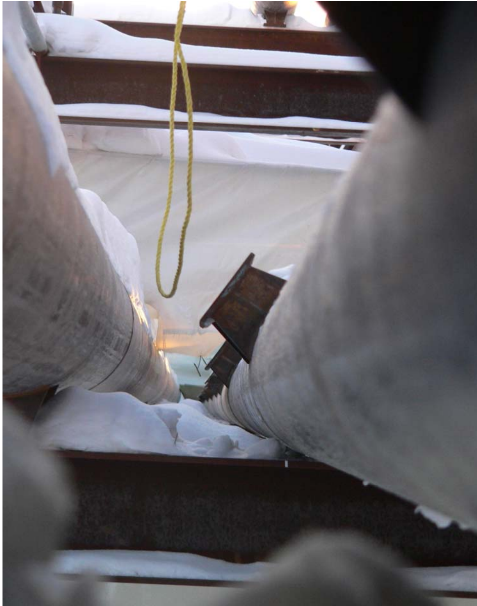
Photograph #8 Looking east; shows the 57 m of 14 inch (355 mm) diameter pipe spool which rolled off the pipe shoes.
