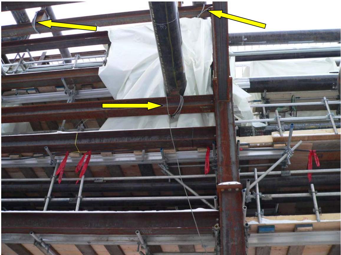
Photograph #10 Shows an expansion loop with various cable lashing used. These were not observed in use on the five pipe spool involved in the incident.
