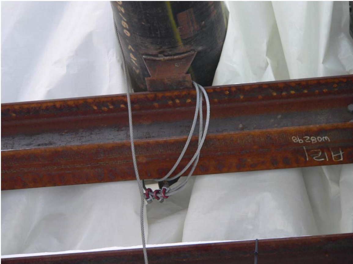
Photograph #9 Shows a method to secure pipe shoes called cable lashing seen being used in the pipe rack #939. These were not observed in use on the 14 inch (355 mm) diameter pipe spool # PW-ABA-14-9353 involved in the incident.
